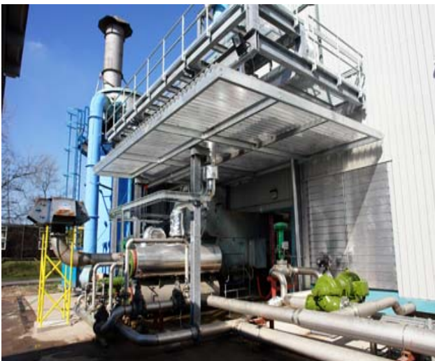
April 2007: Preparations for commissioning programme – compressors
