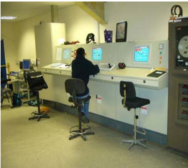
Control Room (Desk designed and built by AIM)
