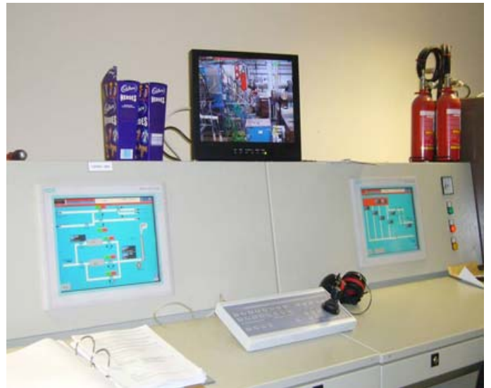
Control Panels with CCTV view of Combustor Room
